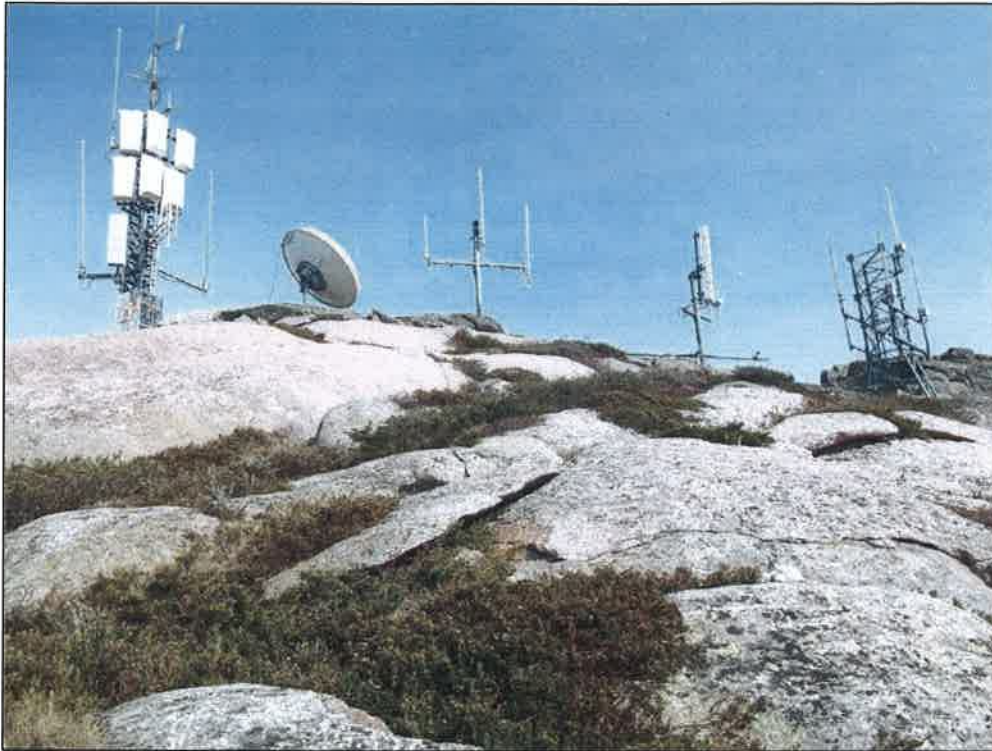
Photo 9: Eagles Nest existing facilities location looking west from top of mountain. Note the 'antenna farm presentation to visitors.
